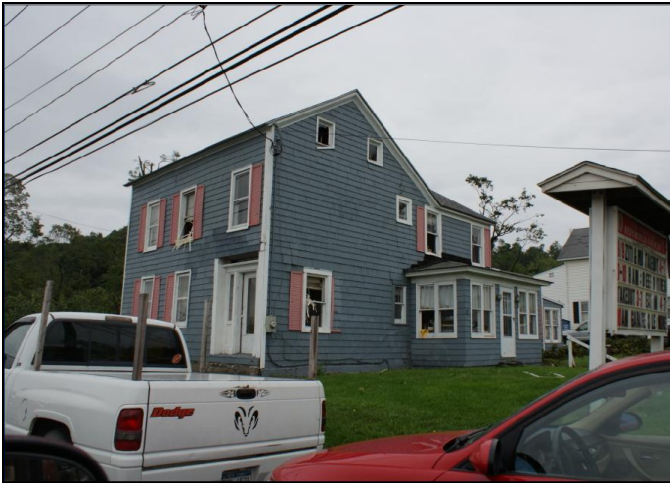
Figure 1: This home along Riverview Rd. in Cranesville had windows blown out, shutters damaged, blinds mangled and in disarray, and some roof damage, from the EF1 tornado. (NWS at Albany Photograph).
