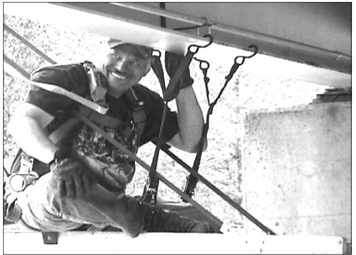
Anchorage Electronics Technicians Dave White (pictured) and Jocelyn Perry installed a depth sensor on the Chilkat River bridge to measure water levels.
