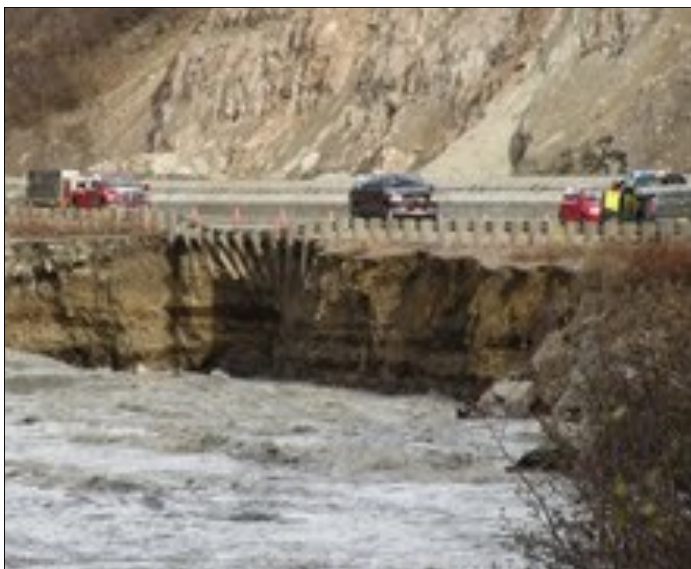
The Nenana River erodes away the Parks Highway at Milepost 239
