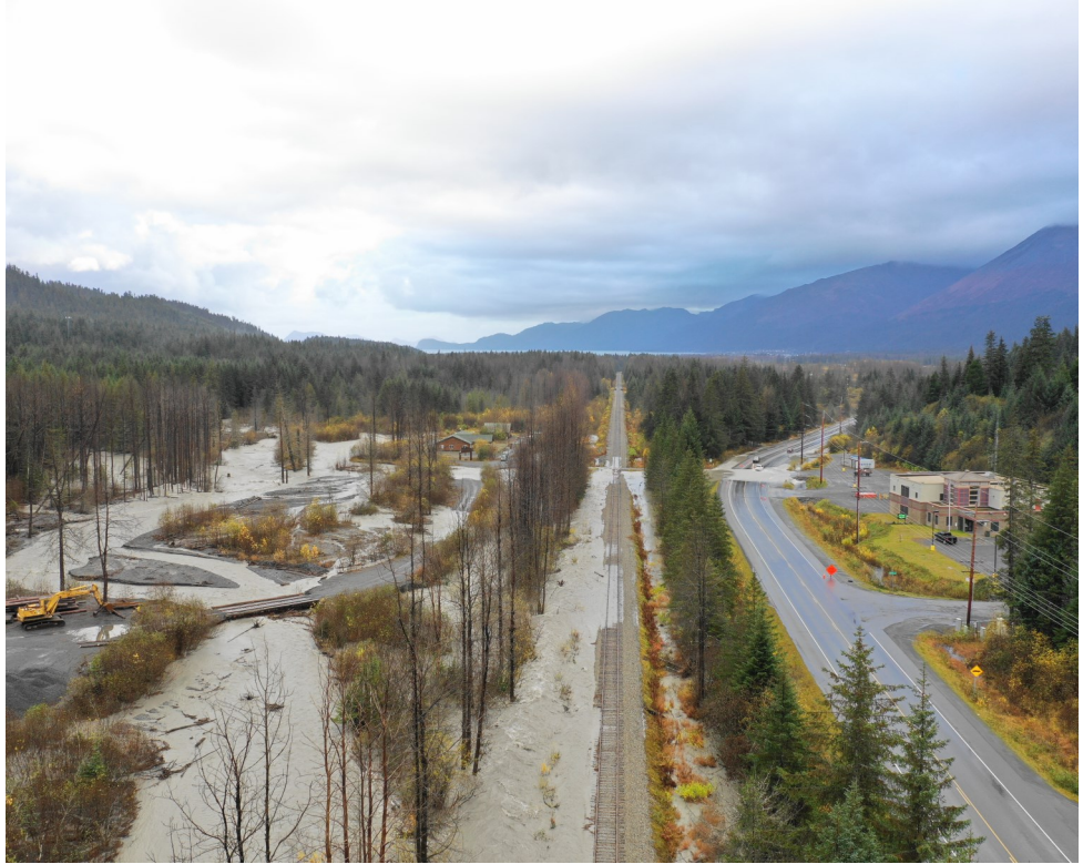
Figure 10: heavy equipment is helping preserve this bridge near Seward by removing gravel from the streambed as it's washed down by heavy rain. Photo courtesy of Alaska DOT&PF.
