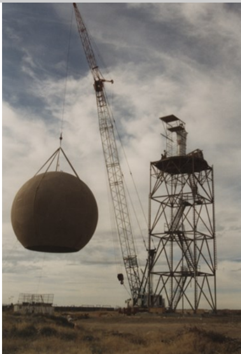
The Treasure Valley radar installed in November 1993. The radar is located a few miles south of the Boise Airport.
