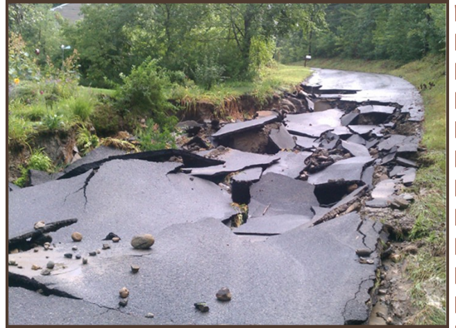
Above: Beebe Road in Monson, MA. had significant damage due to flash flooding on Aug 12th.
