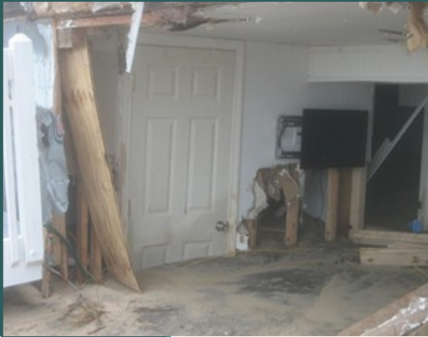
Above: Sand deposited in a home located on Misquamicut Beach, RI.
