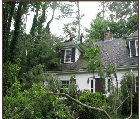
Above: Wind Damage in Wayland, MA on July 3rd. Photo taken by Tom Turner
