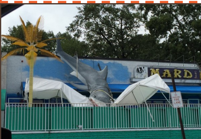
Above: Wind Damage to the Mardi Gras in Cranston, RI. Picture by John Buco.
