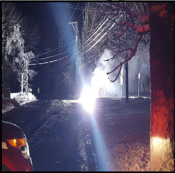
Above: Downed Power Lines in Acushnet, MA - Photo: Ed Caron-KA1RSY - Acushnet EMA
