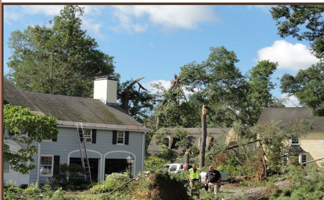
Above: Damage in Concord, MA. Photo courtesy of NWS Taunton Amateur Radio
