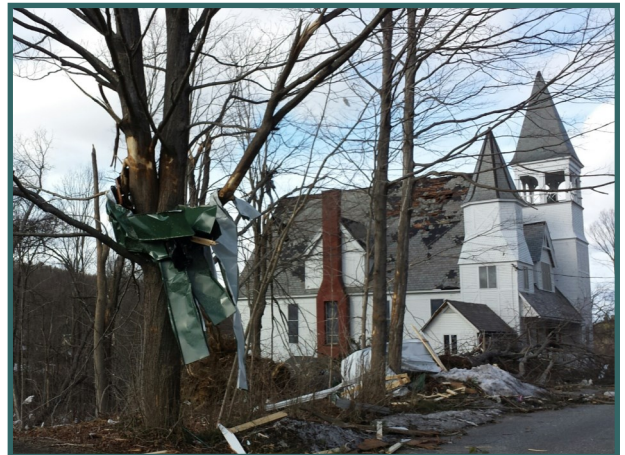
Above: Tornado Damage in Conway, MA.
