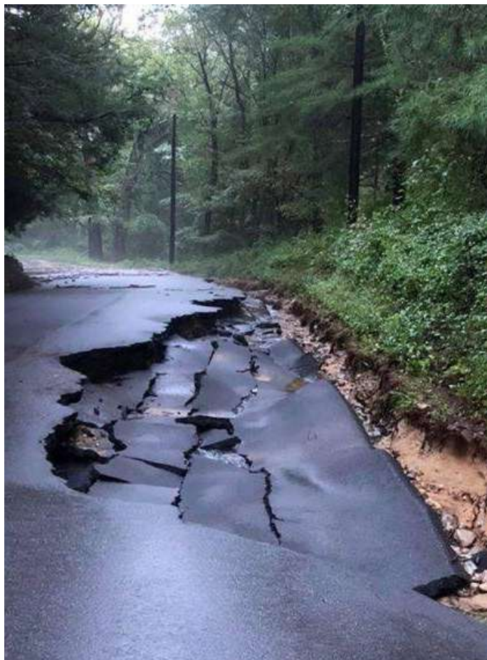
Road Washout on Station Road in Scotland, CT Photo by: KC1CVU-Rusty Lanzit
