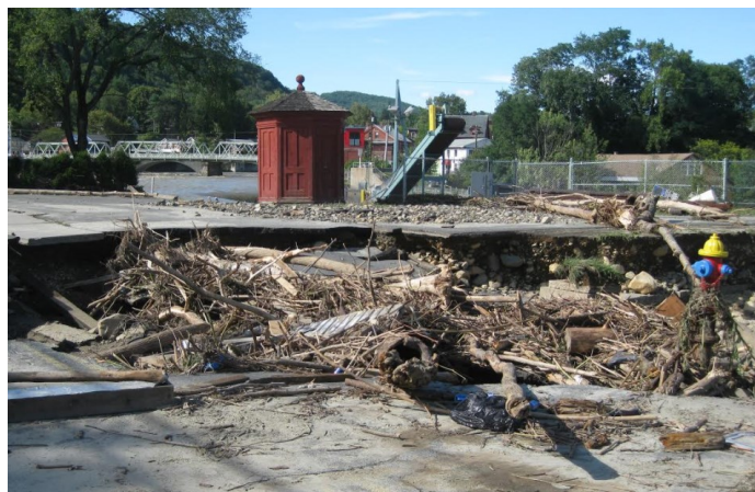
A roadway torn up by flood waters in Shelburne Falls, MA
