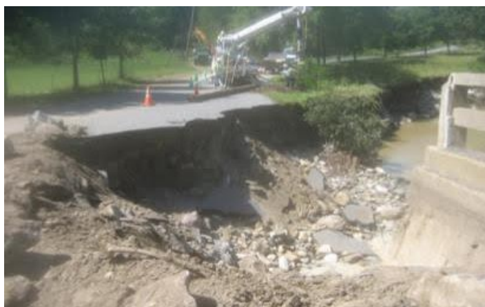
A washed out bridge on the West Branch of the North River in Colrain, MA
