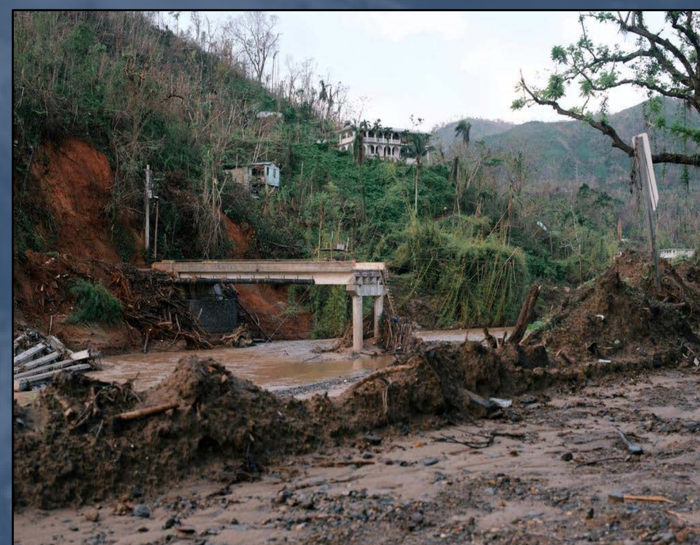
Collapsed Bridge in Utuado (Eliud Echevarria, FEMA)
