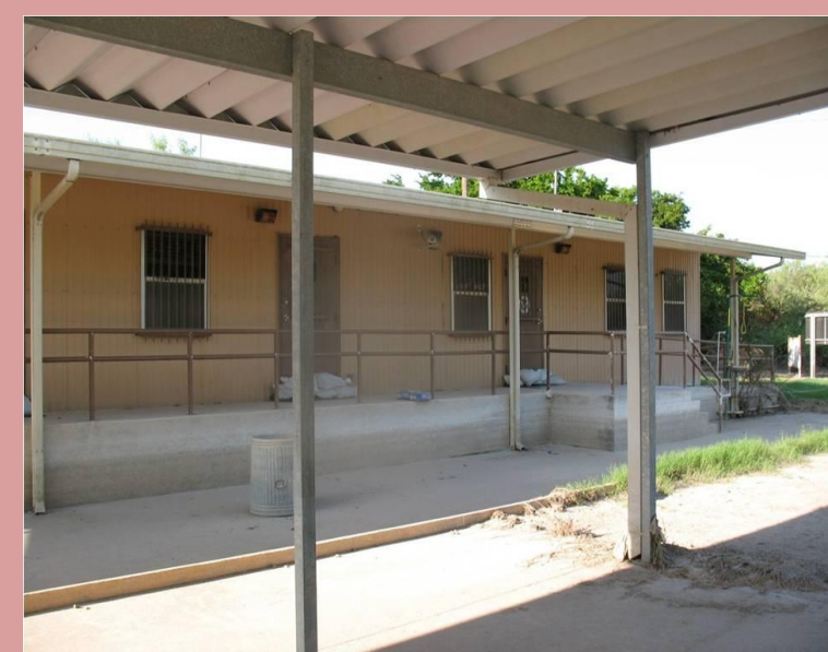
U.S. Customs office damaged in Los Ebanos, Texas
