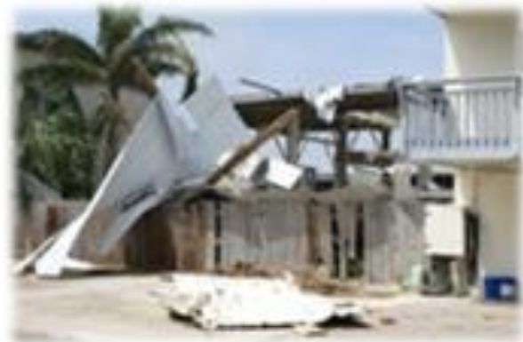
Figure 4. Photo of damage to apartment complex in Port Isabel, TX, taken on 24 July 2008, one day following Hurricane Dolly. Descriptions in Figure 3 for apartment building damage were nearly identical to what's shown.
