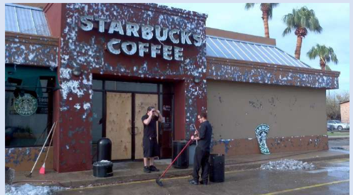
Photo of damaged storefront in McAllen courtesy of National Weather Service Brownsville Storm Survey Team
