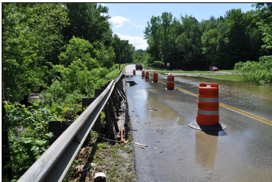
Flood damage to road. Photo Credit: NOAA/NWS Burlington
