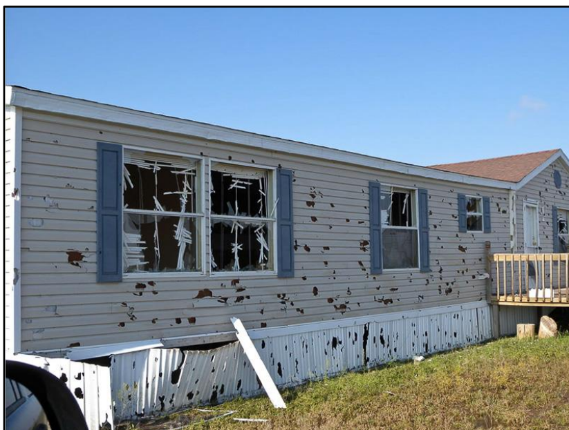
Hail damage to a home. Photo Credit: NOAA/NSSL
