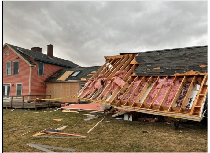
Figure 6: This picture was taken north of Painter Hill Road where the most significant damage associated with the short-lived tornado occurred. Shingle damage to both the north and south facing side of the house was noted. In addition, an attached garage was removed from the foundation and thrown 10 feet where it collapsed. This damage is what led the survey team to rate the tornado as a high end EF-1.
