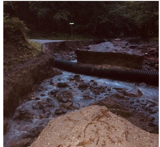
Figure 4: Road washout in Waitsfield, VT. Courtesy of Waitsfield Emergency Management.
