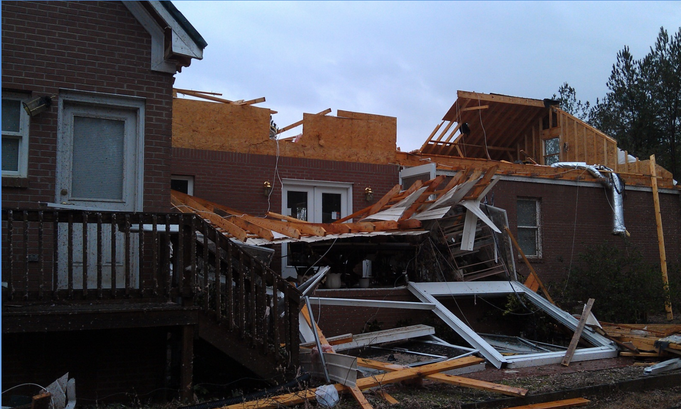
Damage associated with the tornado near Wagener
