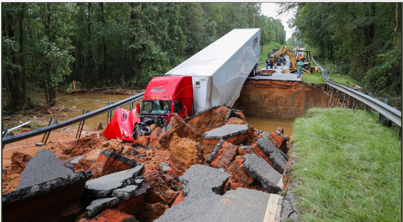
Hwy 145 in Chesterfield County SC washed out. (Photo courtesy Chesterfield Co. Sheriff)
