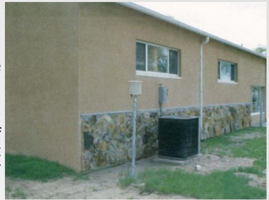
Temp Sensor right next to HVAC unit which would give a bad reading!
