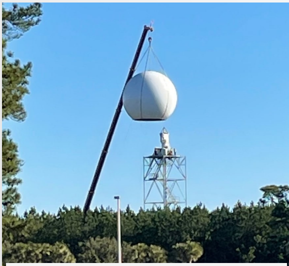
The crane lifts the dome protecting the radar to replace the pedestal.
