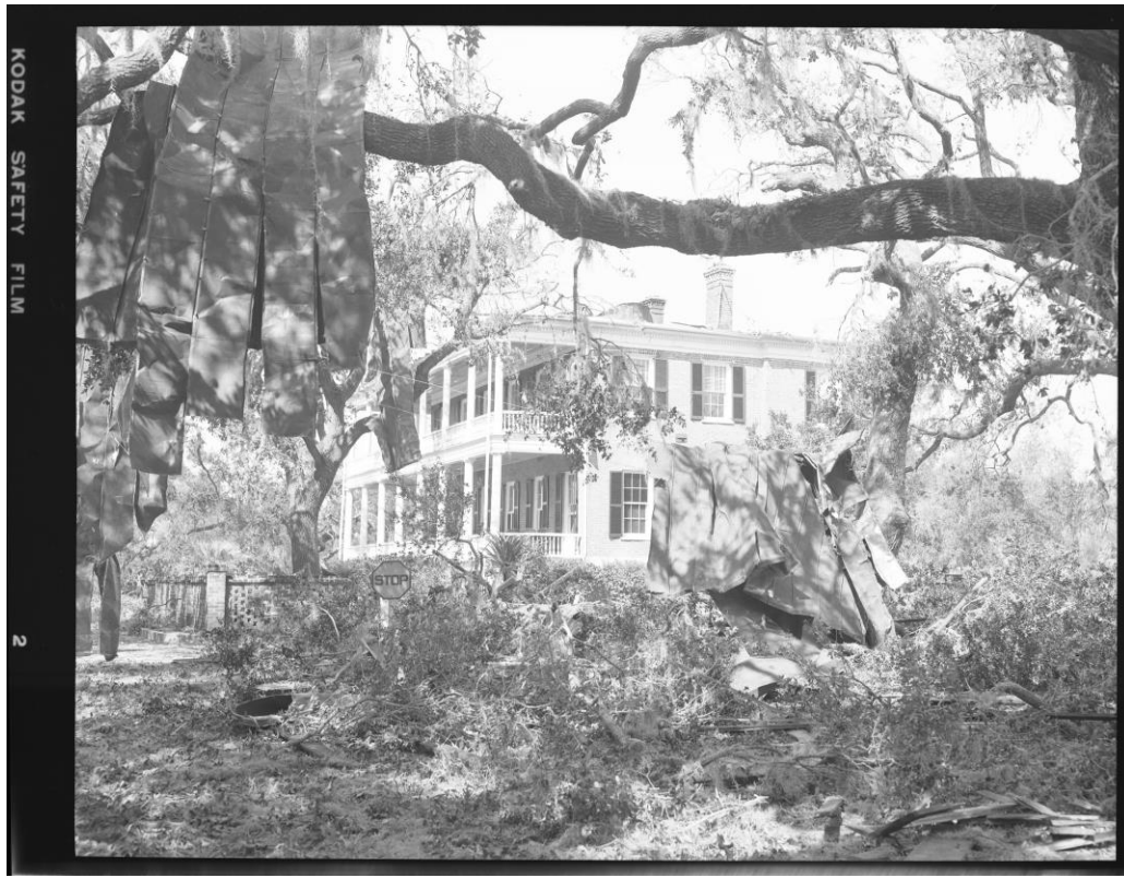
Damage to the Edward Means House from Hurricane Gracie. Image courtesy of Beaufort County Library, SC.
