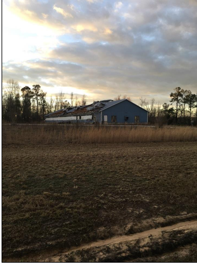
Storage building roof damage from Screven County, GA EF-0 tornado near Buttermilk Road on January 21.
