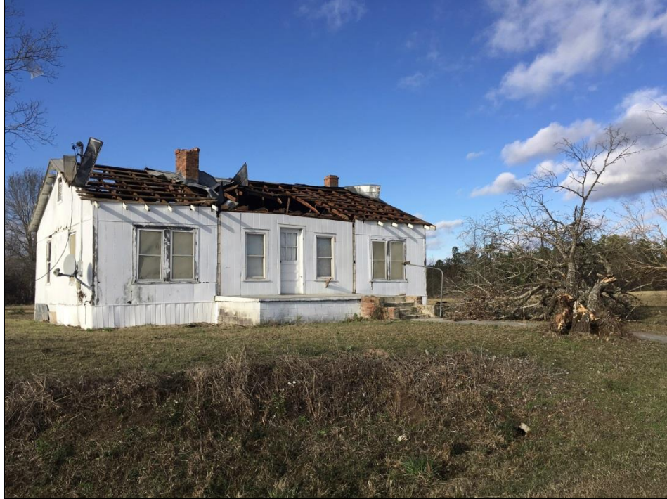
Damage caused along Friendship Road by the second Screven County, GA tornado on January 21.
