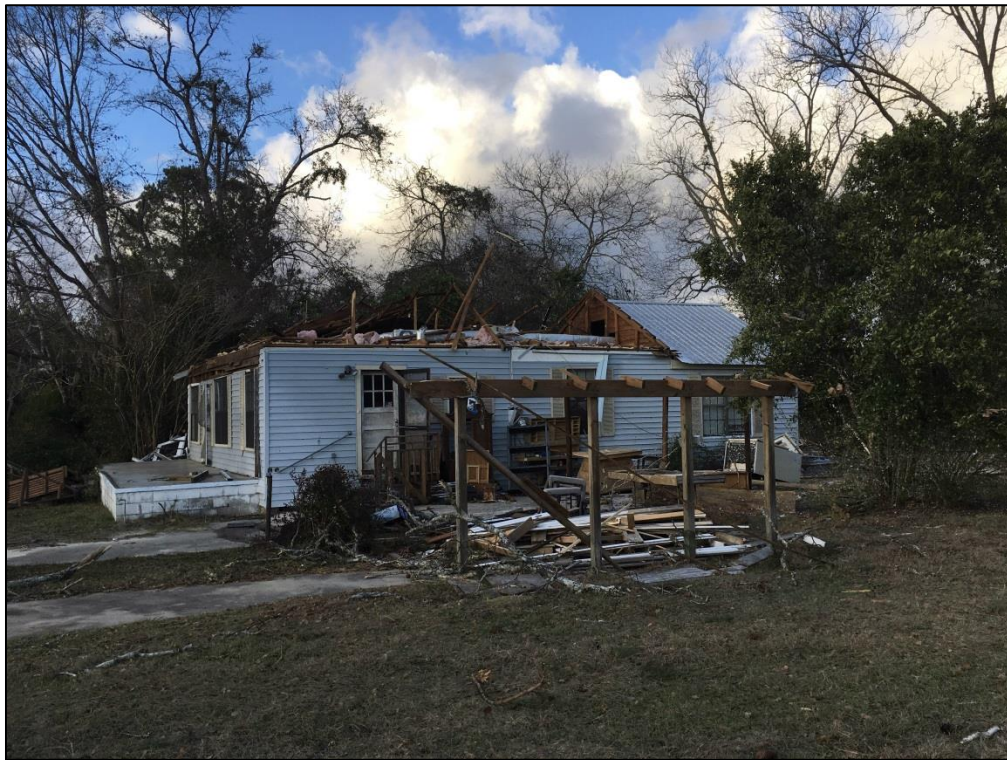
EF-1 damage produced along McBride Circle by the second Screven County, GA tornado on January 21.
