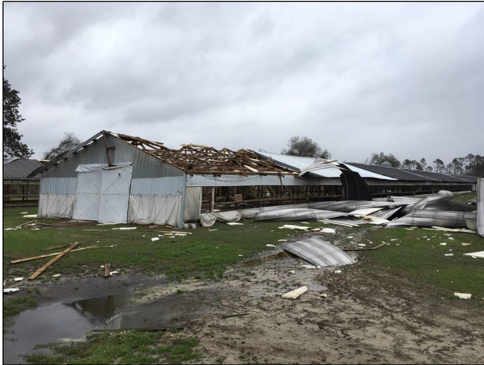
Damage from Tattnall County, GA EF-0 tornado near State Route 178 on January 21.
