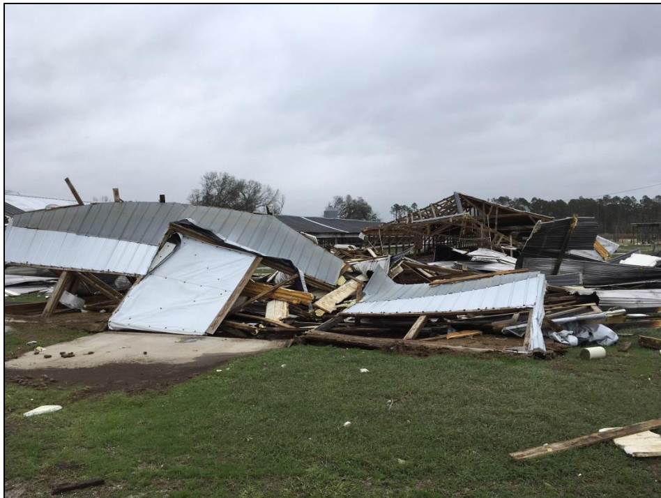
Damage from the Tattnall County, GA EF-0 tornado near State Route 178 on January 21.
