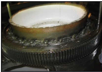
Damaged Bull Gear
