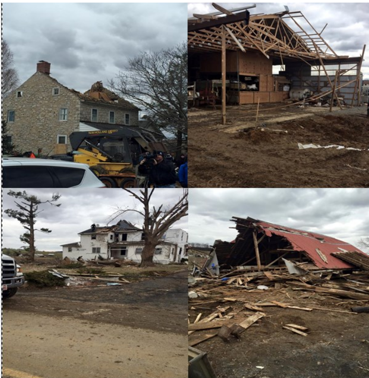
Figure 3. The top left image is of a house that had its roof completely blown off. The top right image is of a machine shed that sustained heavy damage. The bottom left image is of a house that had the roof blown off and windows blown out. The trees were almost completely delimbed. The bottom right image is of a shed that was completely destroyed.
