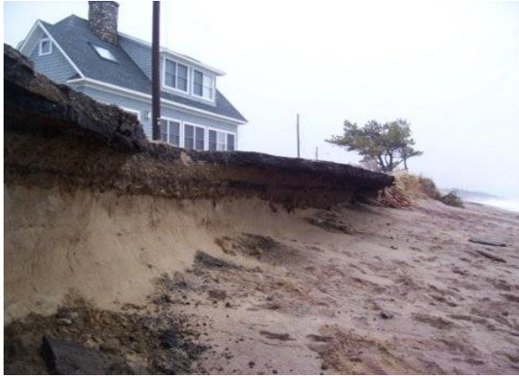
Figure 5. An example of splash-over damage in Saco, Maine during the Saint Patrick’s Day, 2007 storm caused by the battering of ocean waves.
