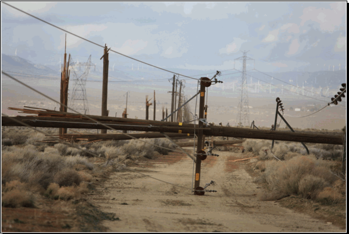
Wind damage from high winds up to 80 mph on March 7th in the Kern County desert. Images courtesy So Cal Edison.
