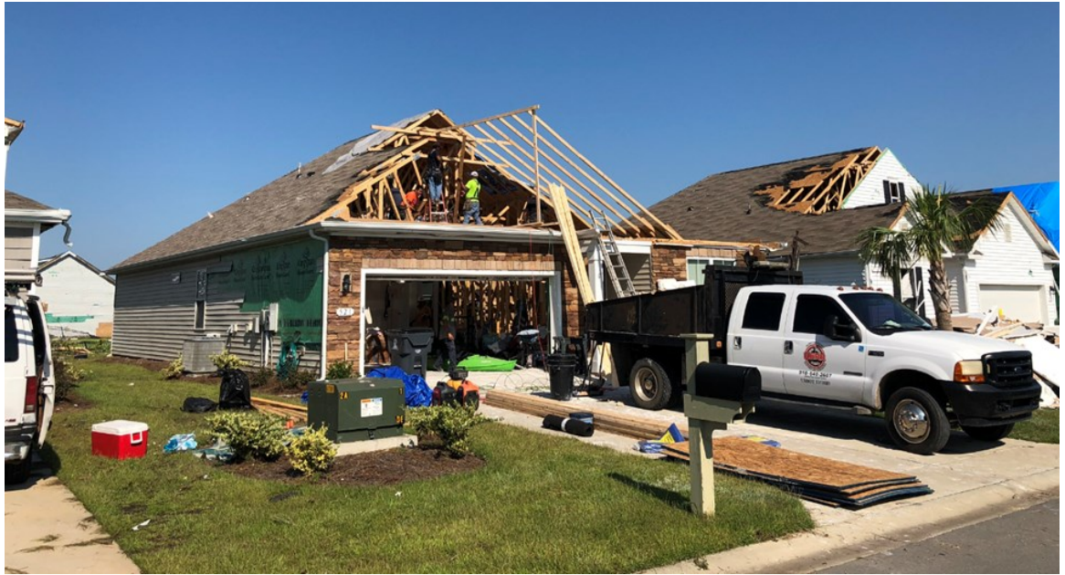
NWS meteorologists conducting a storm survey took this photo of damage to homes in Carolina Shores, Brunswick County, NC, after the early morning tornado of September 5, 2019.
