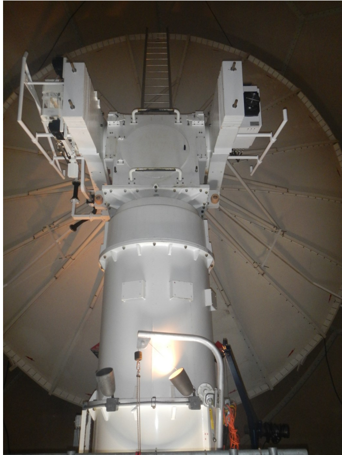
A view of the NEXRAD Pedestal, with the RF Pallet on the right and AME on the left.
