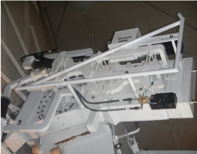
The RF Pallet, part of the Dual Polarization upgrade. This component splits the main transmitted pulse into horizontal and vertical components.
