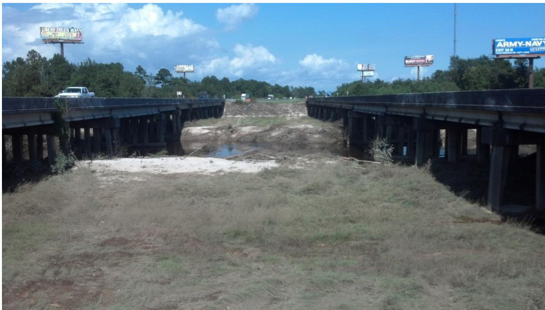
423 424 Figure 16. Wolf River floodplain between the eastbound and westbound bridges of I-10. 425 Widespread tree/brush damage was noted along with scouring of the overbank areas. 426 427
