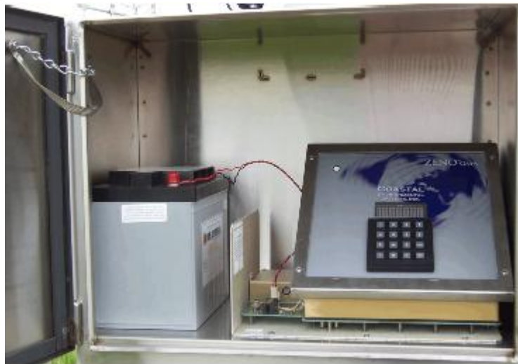
Figure A-16. Data Logger Box
