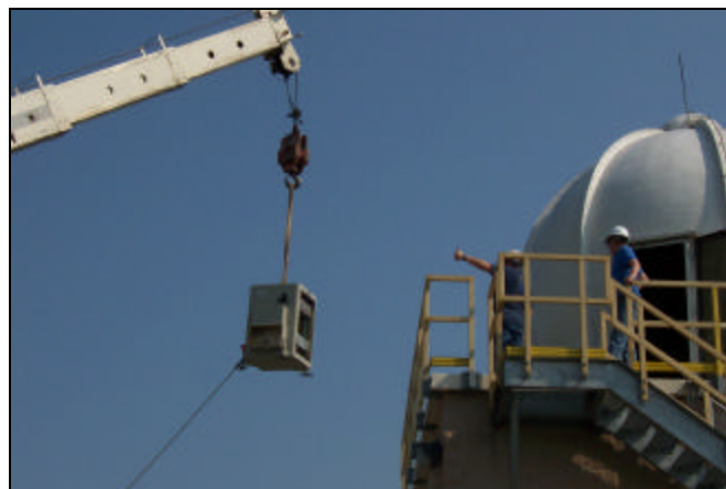
A crane lifts the new equipment to the dome of the upper air shelter
