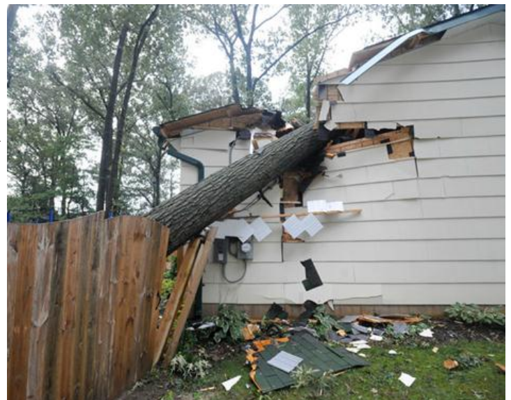
Storm Damage in Severna Park, MD
