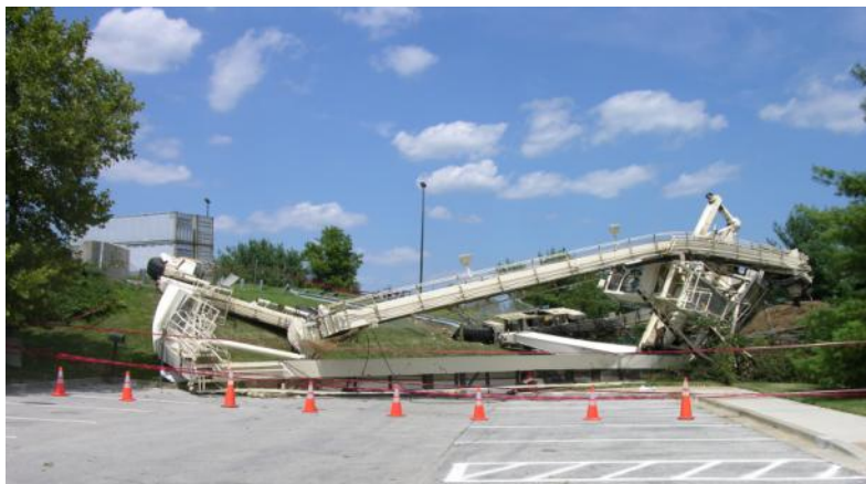
Collapsed crane in Montgomery County. Photo Courtesy: Montgomery County Emergency Management
