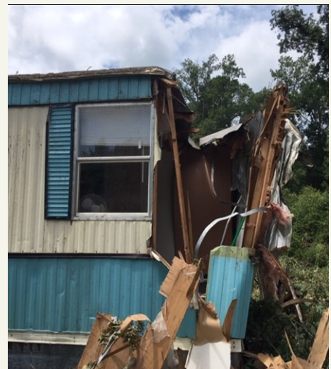
Tornado Damage in Jamesville
