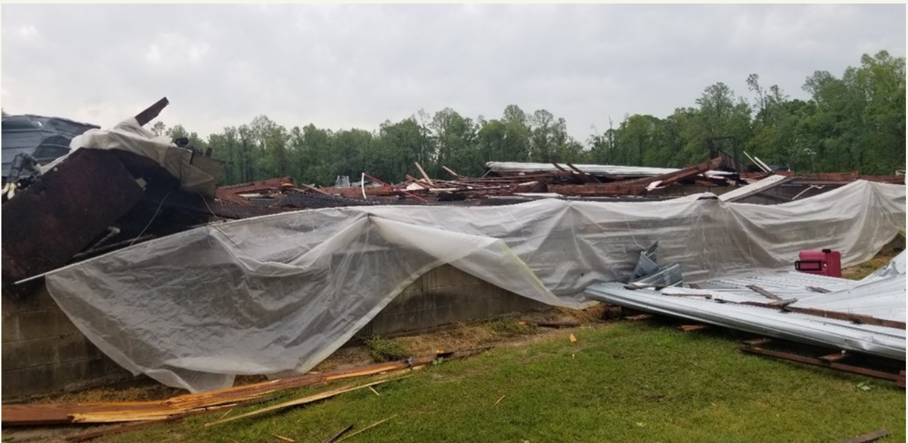
EF-1 tornado destroys farm in Haws Run on April 13, 2020.
