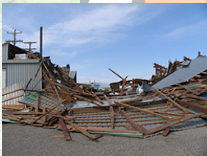
Downburst damage south of Interstate - 84, May 2006
