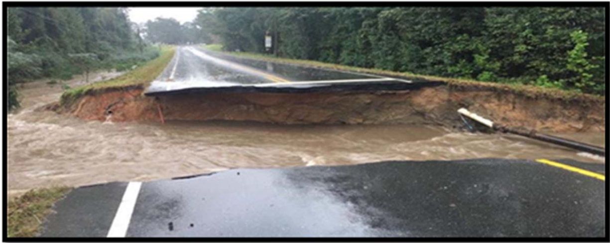
Figure 6: Washed out road near Fayetteville, NC. Source: Reuters
