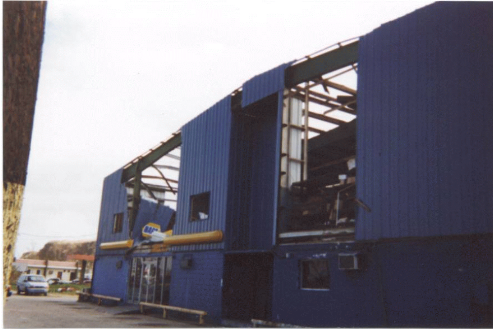
Damage to a commercial warehouse across from the Governor's Complex in Adelup, Guam. (NOAA)
