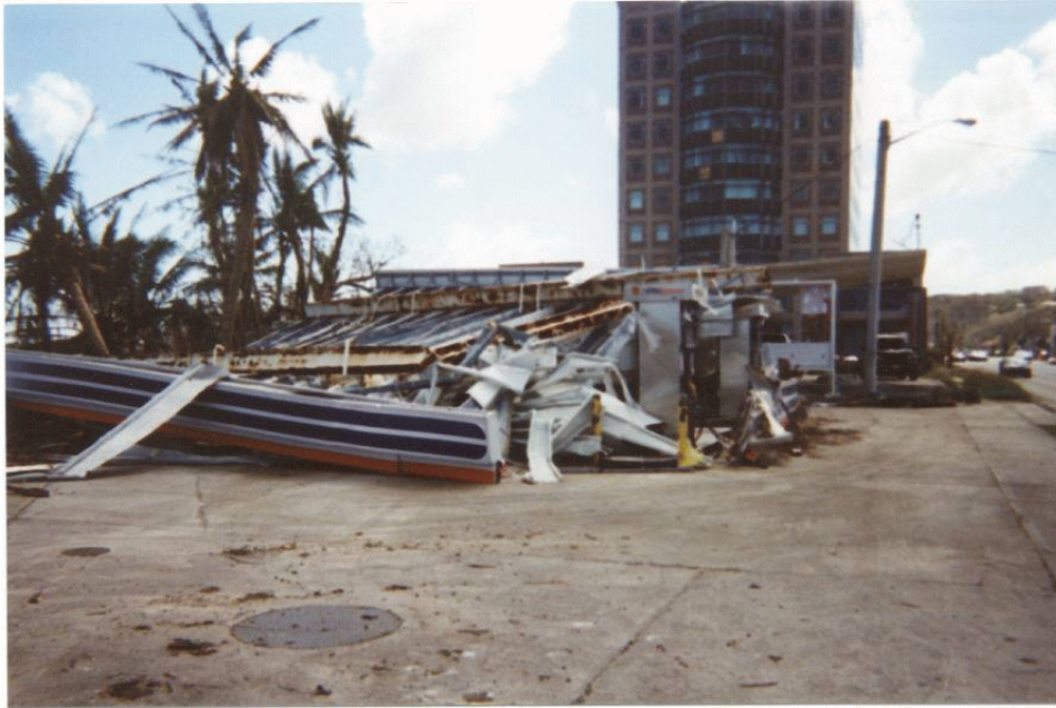
Wreckage of a gas station along Route 4 in Agana, Guam. The Bank of Guam is in the background. (NOAA)
