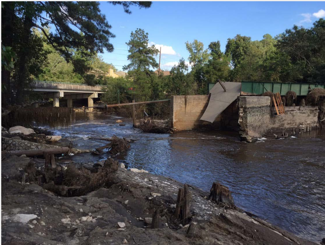
Figure 18: Gibson Pond Dam on Twelve Mile Creek in Lexington, SC, fails.
