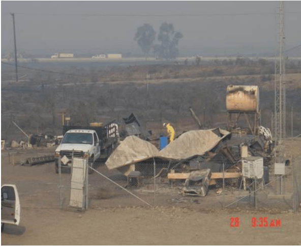
Picture 2. Destroyed office and storage trailers at Upper Air Facility. Courtesy of WFO San Diego.
