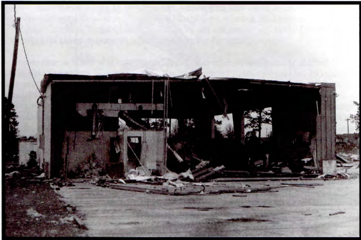
Figure 1-4. Damaged Industrial Park from the Ground. (Photo courtesy of Kevin McCarthy.)
