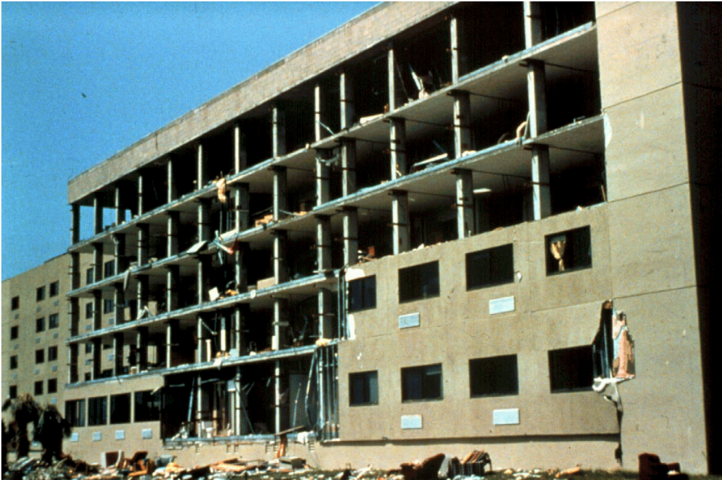
Intense winds associated with Andrew caused the shearwall to fail on the lee side of this multifamily structure
