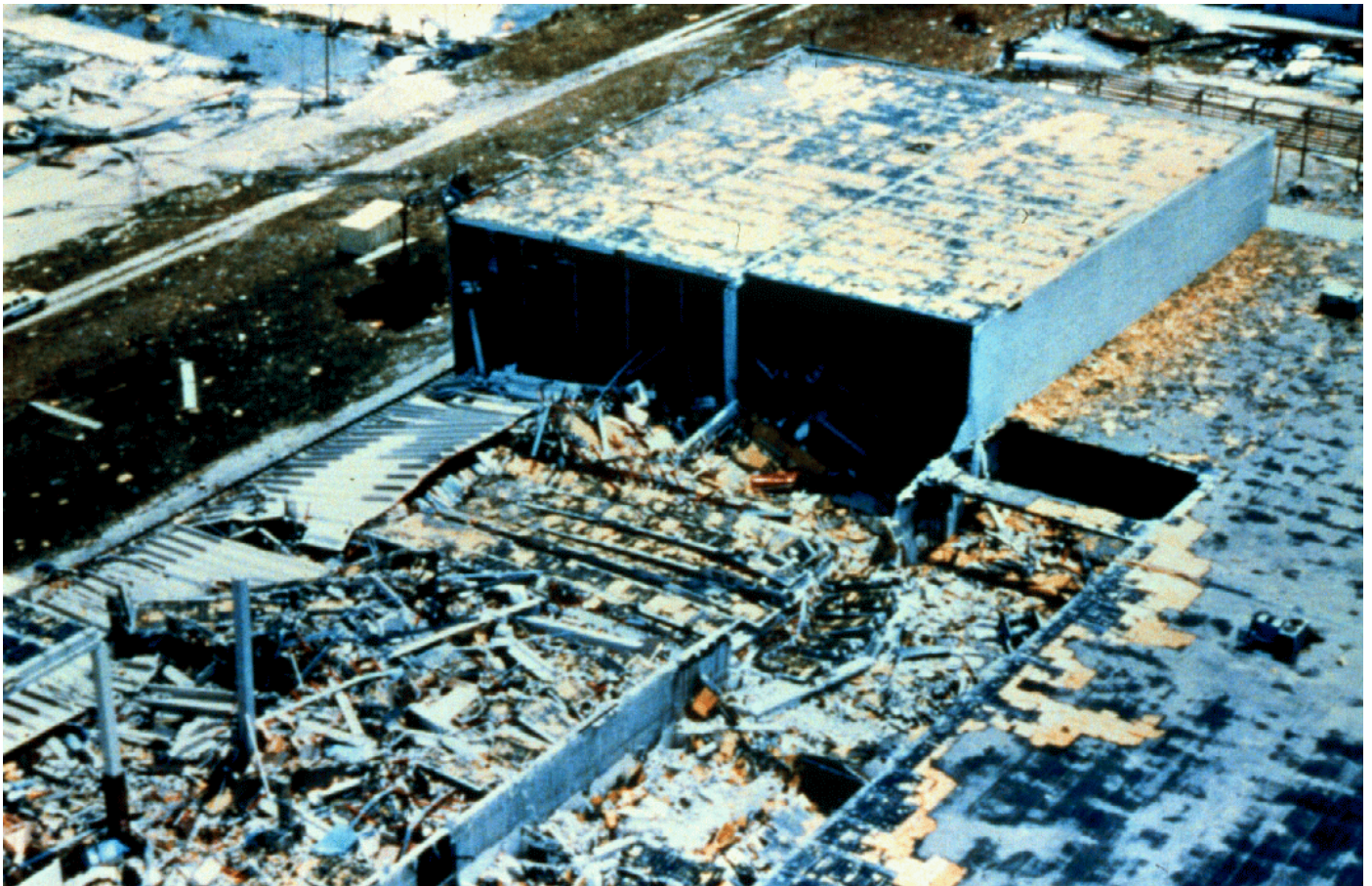
Levitz furniture warehouse, west of Whispering Pines, Florida, shows extensive wind damage.
