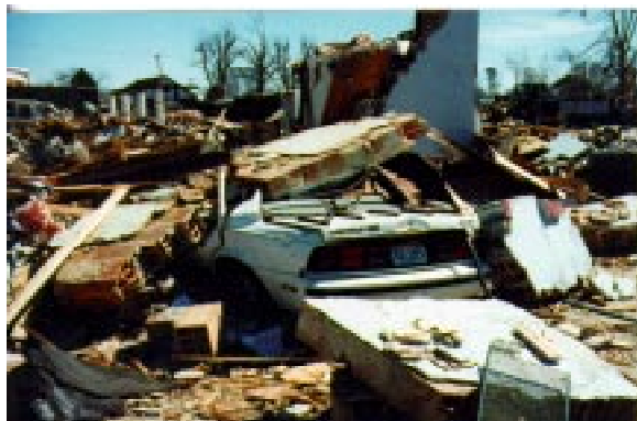
Substantial buildings, such as these brick and block buildings, were completely destroyed from the devastating tornado that struck within a few blocks from downtown Arkadelphia. Courtesy of Chris Smith, NWS Southern Region.
