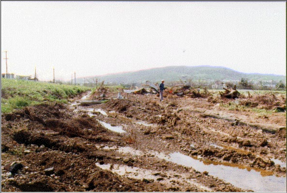
Figure 1-20. Eroded streambed alongside airport on Culebra. (Photo courtesy of Don Wernly)
