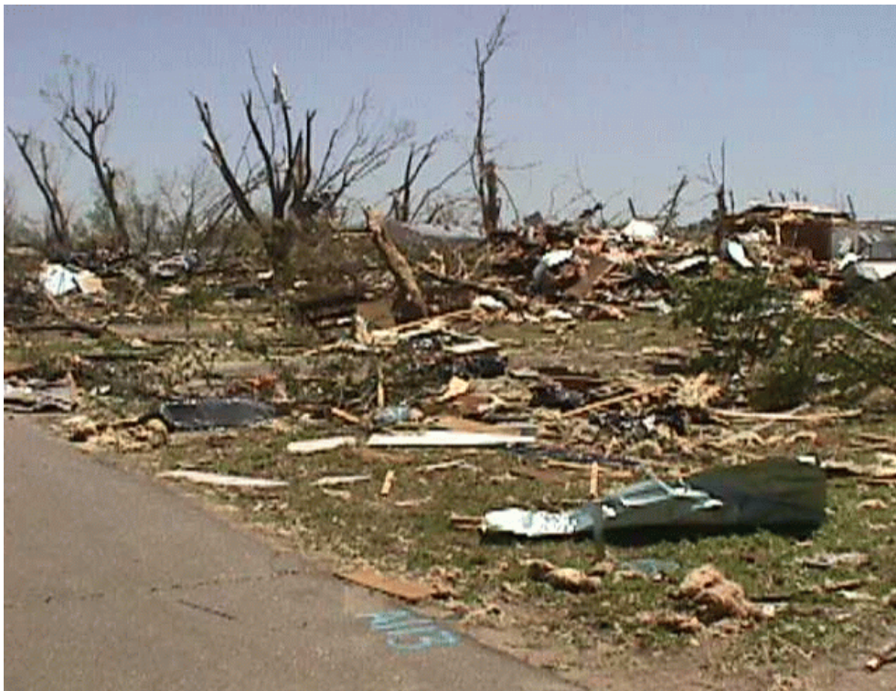
Devastating tornado damage in the small community of Haysville, south of Wichita, Kansas. (Photograph courtesy of John Ogren, NWSO Wichita, Kansas)
