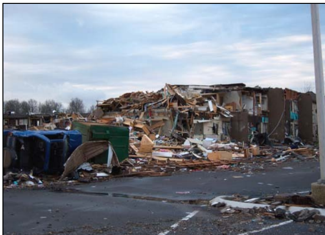
Figure 10. Damage to dormitories at Union University in Jackson, Tennessee. Courtesy of WFO Memphis.
